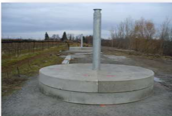
PS5000 DropNGo Ballast as installed
