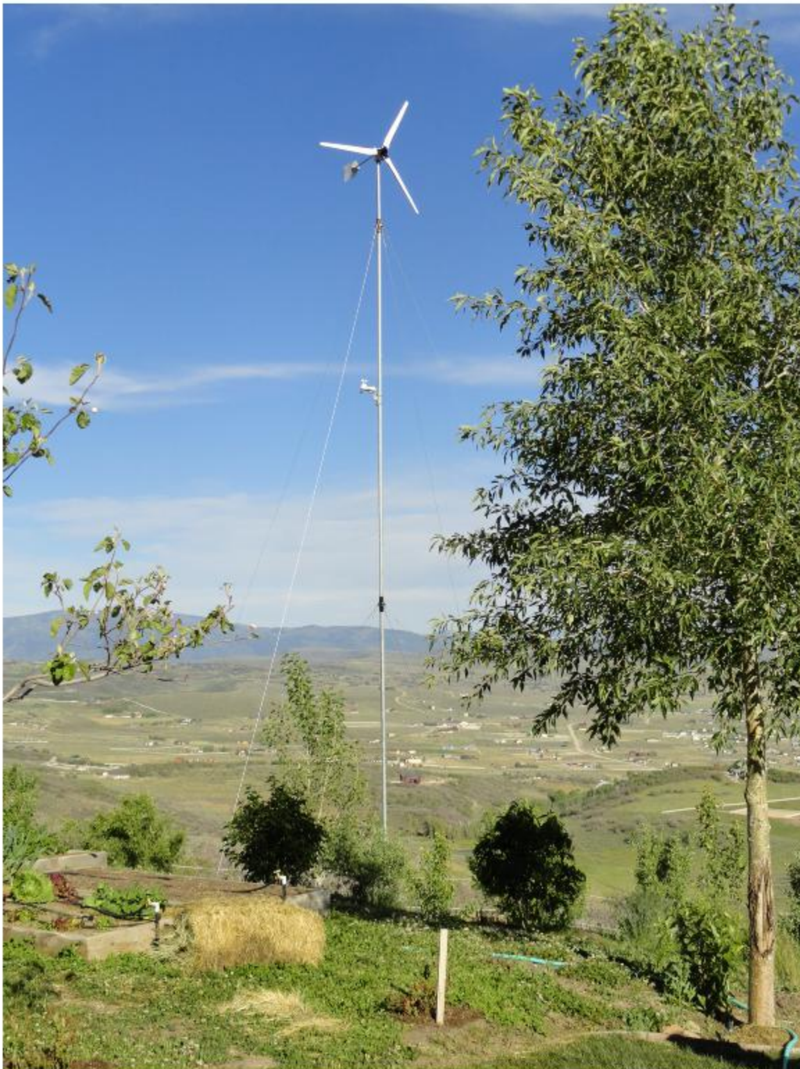
Properly installed wind turbine generator using a guyed tilt tower and weather station.
